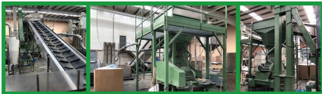
Heathland's pretreatment installation
